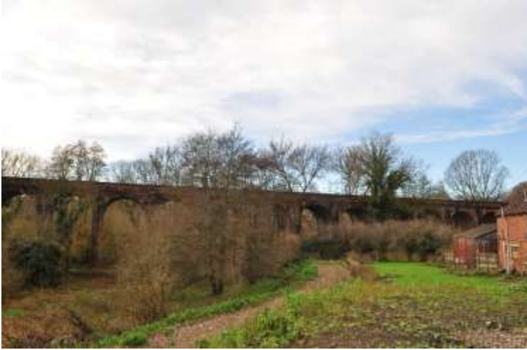
View 6c – Broad span of viaduct arches from public footpath WT192 looking west
